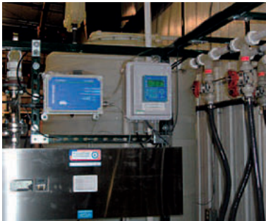
770MAX and 5000TOC sensor connected to water system.
